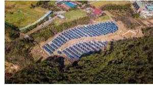
S-18 CS Takayama-shi Power Plant 1.0MW
