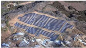
S-11 CS Minano-machi Power Plant 2.4MW
