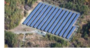
S-14 CS Koriyama-shi Power Plant 0.6MW
